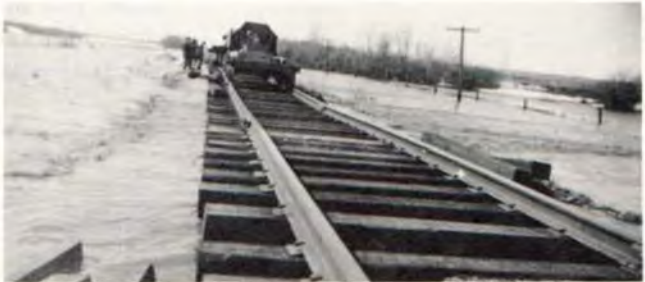
Flood of 1956 (S.E.-22-56-17-4). Extensive damage was done to the railway.
